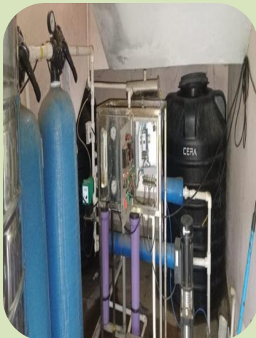
R.O. WATER PLANT
